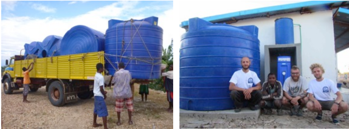
Figures /15/16. Rain-water collection tanks manufactured for installation at the Hospital in Fotadrevo
