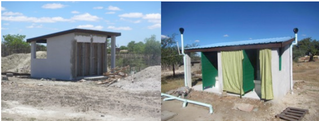
Figure 13/14. The toilets and showers for guest and family members of patients under construction
