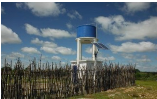
Figure 3. New water well with tower with solar panel for the submersible pump.
