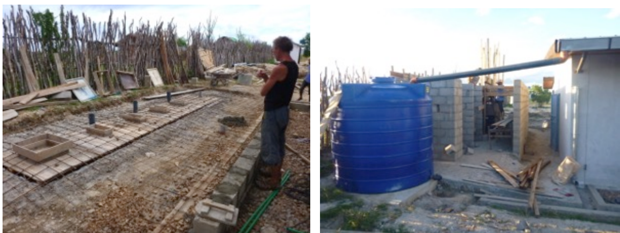
Figures 9/10. The toilets and showers for patients outside
